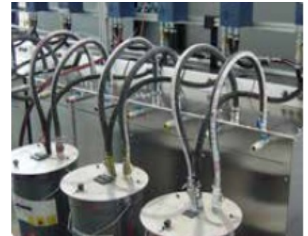
Automatic Washup System
